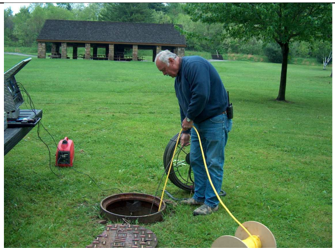
Pennsylvania Rural Water Wastewater Training Technician Kurt McFadden helps Chuck Wagner of Keystone State Park locate a sanitary sewer line break.
